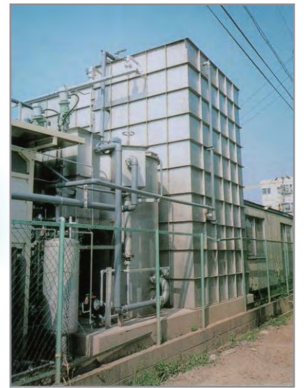
Stainless treatment tank
